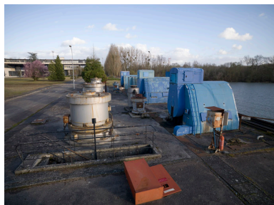
Stations de pompage. Phot. Philippe Ayrault IVR11_20087700455NUC4A
