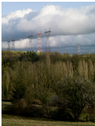
Pylones lignes haute tension. Phot. Philippe Ayrault IVR11_20087700483NUC4A
