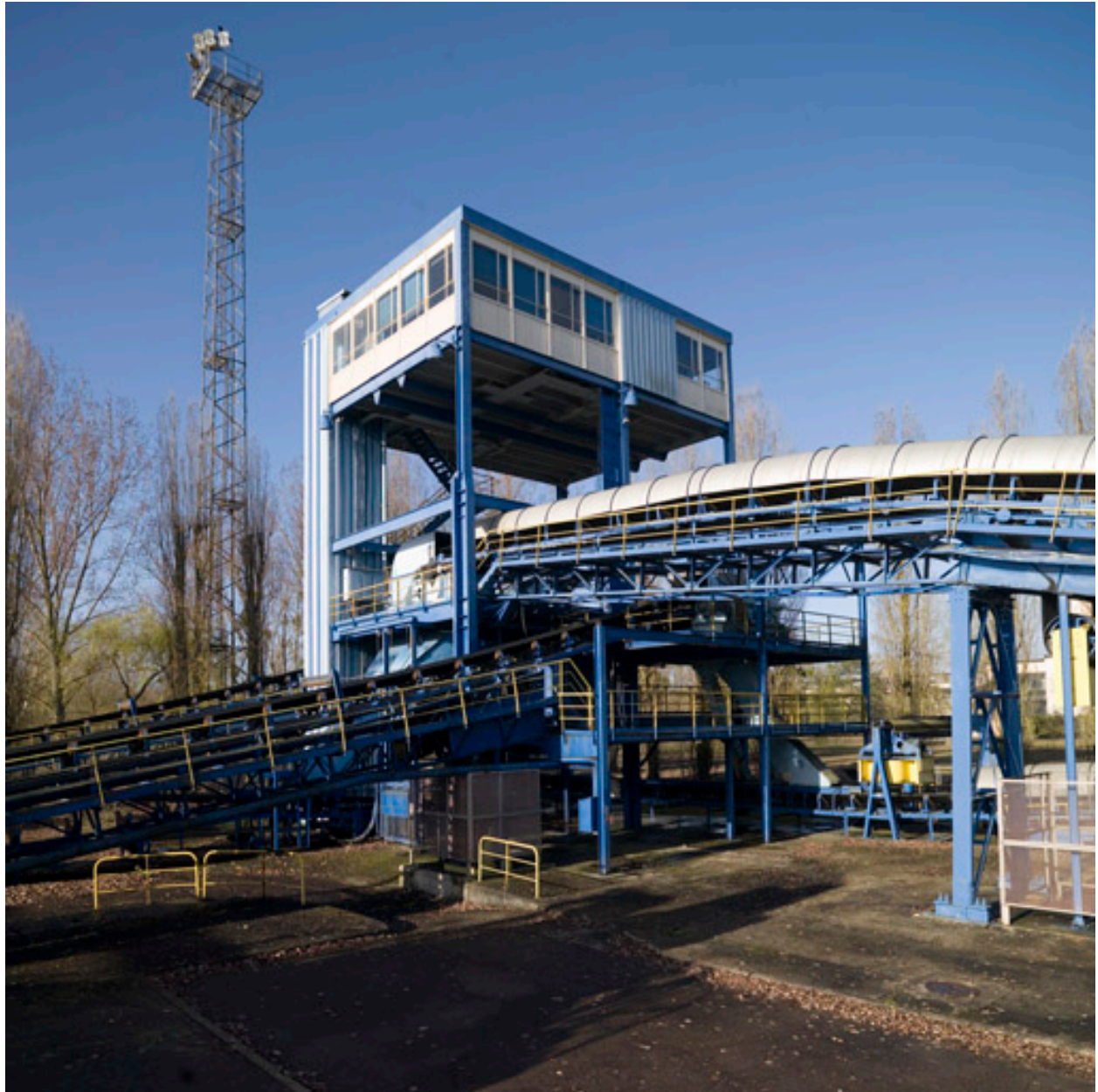
Parc a charbon. Manutention.
