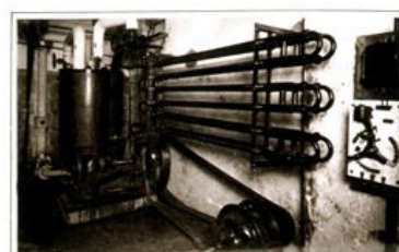
INSTALLATIONS FRIGORIFIQUES (Pompe 10 000 kg/cm 2 )
